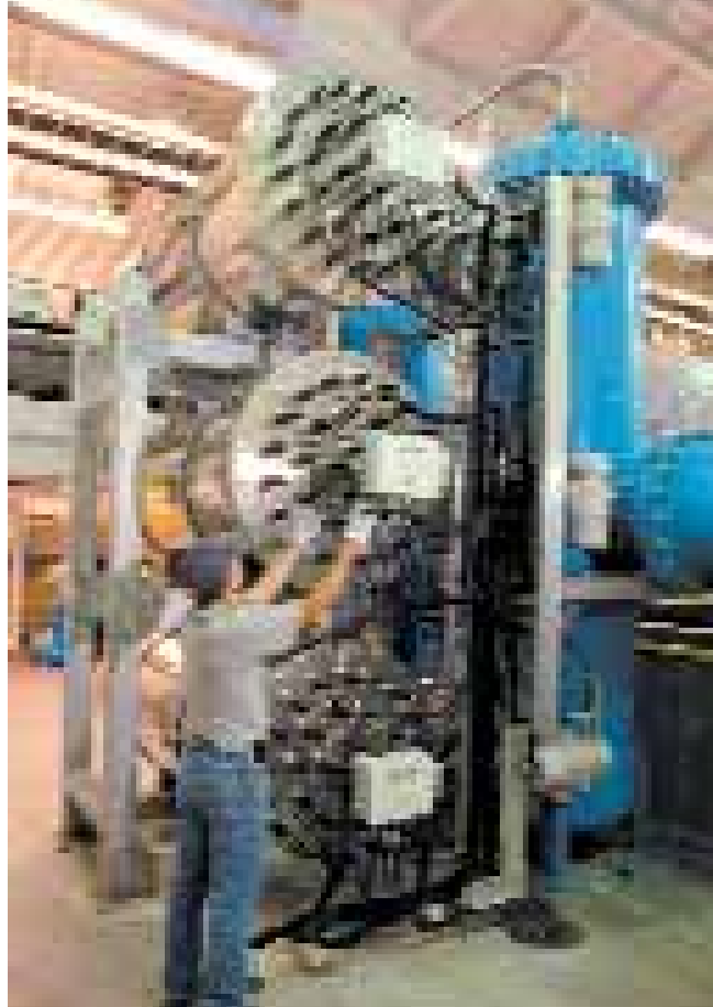
Chief operator, David Carlson, checking UV reactors
